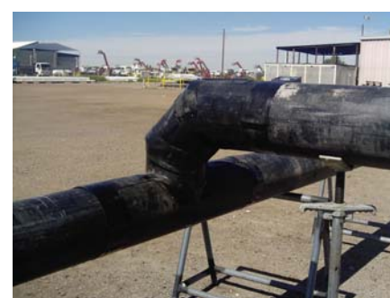
Apply heat shrink to complete fitting
