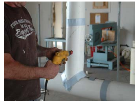
Drill 1" hole on each side for foam and apply tapecoat to seams
